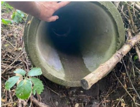
Figure 5: Photograph of discharge pipe onto the Subject Farm
