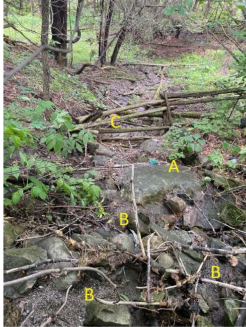
Figure 12: culverts and stormwater infrastructure feeding the concourse showing damage
